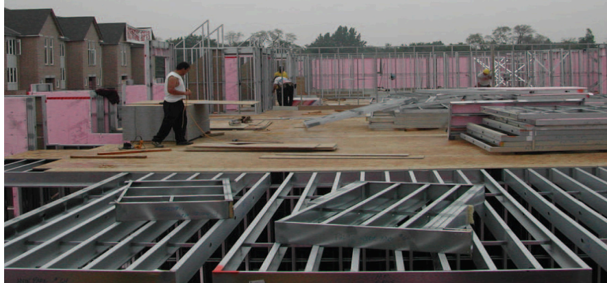
Hyde Park Condominiums (Zentil): Genesis™ steel panels and roof trusses made from light steel framing contribute significantly to meeting several of the prime building considerations - quality, lightweight and speed of erection.
